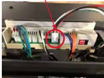
New Wiring Harness
